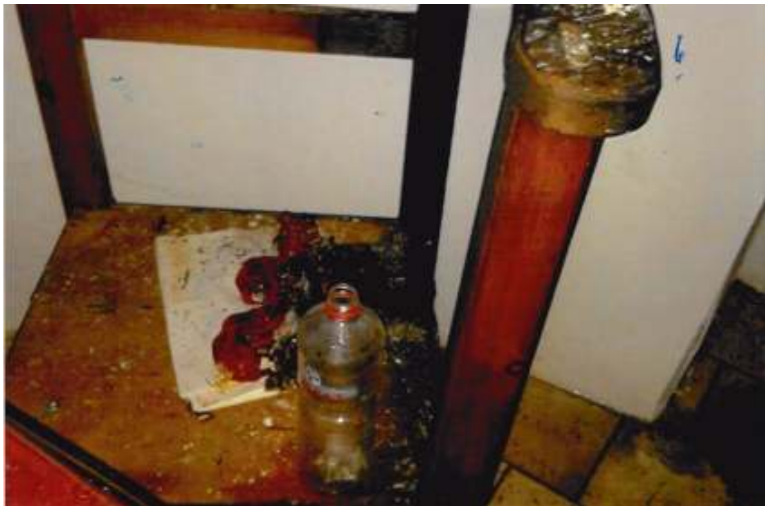
Damage caused by the fire
