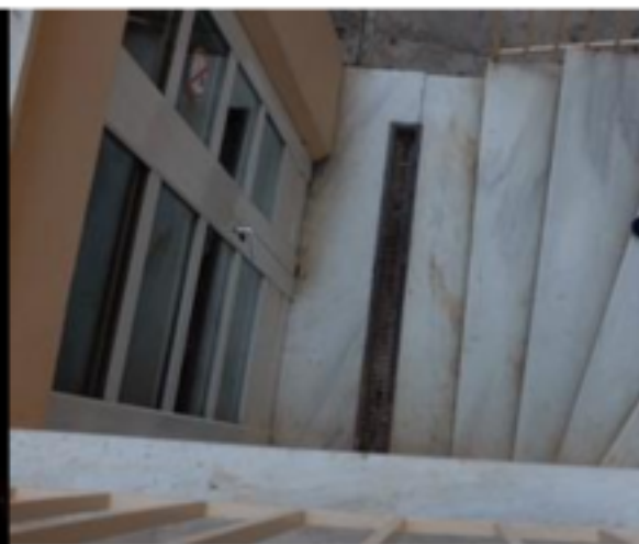
The metal grating which was lifted and carried for several meters and was used in the end as a lever for breaking the door
